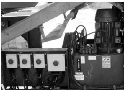
Integrated electric powerpack for bucket wheel speed adjustment
